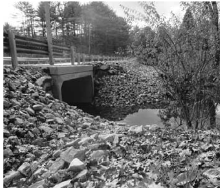
Photo of completed Shorey Bridge project (Photo courtesy of Jon St. Pierre)
