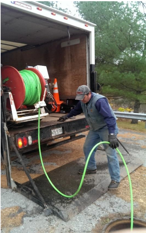
Jeff Curtis of Interstate Septic jets a pipe from Manhole 99 on Four Rod Road on October 28, 2014
