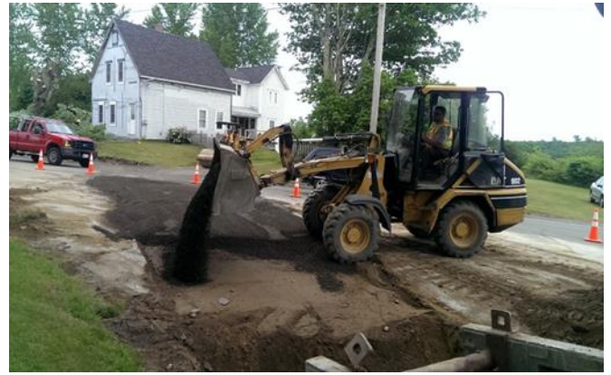
Jacob Bryant of George C. Hall & Sons Backfills a pipe crossing Route 1 June 25, 2014
