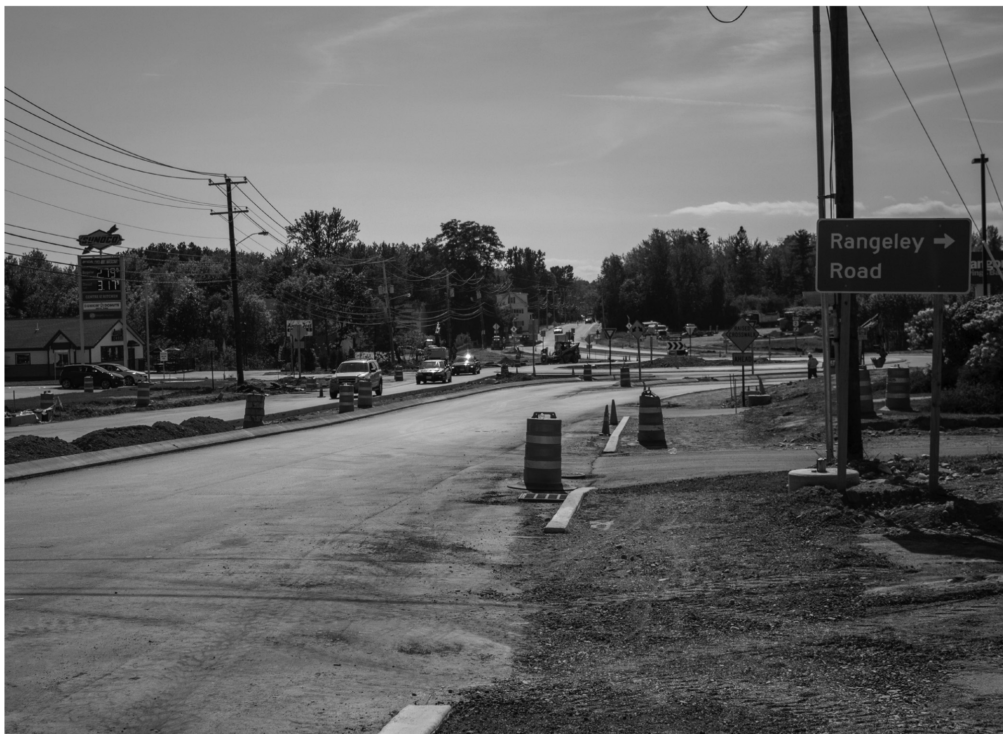
The rotary at Rangeley Road is still under construction, but making a difference in students' commutes to campus.
