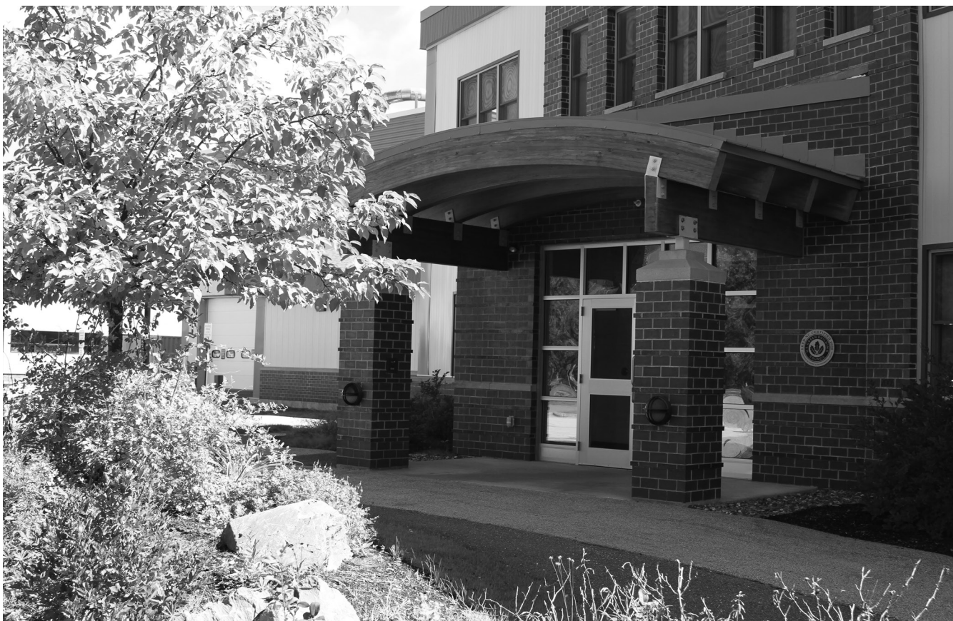
Construction is underway on the latest addition to the Advanced Structures and Composites Center.
