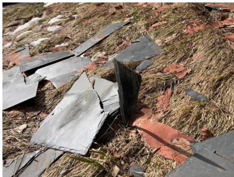
Figure 120. "Site-work: High winds cascaded slate papering and shingles driving one into the ground."
