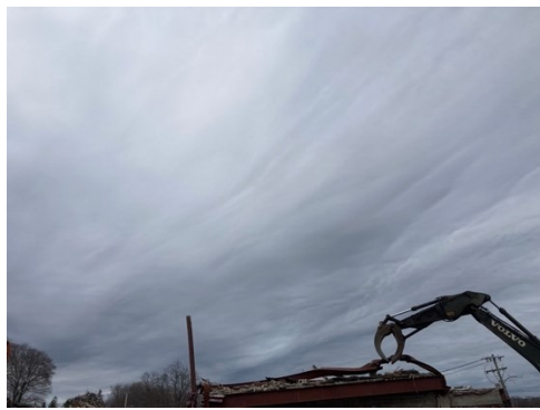
Figure 119. "Site-work, silhouette of excavator arm delicately lifts steel I-beam out from position."
