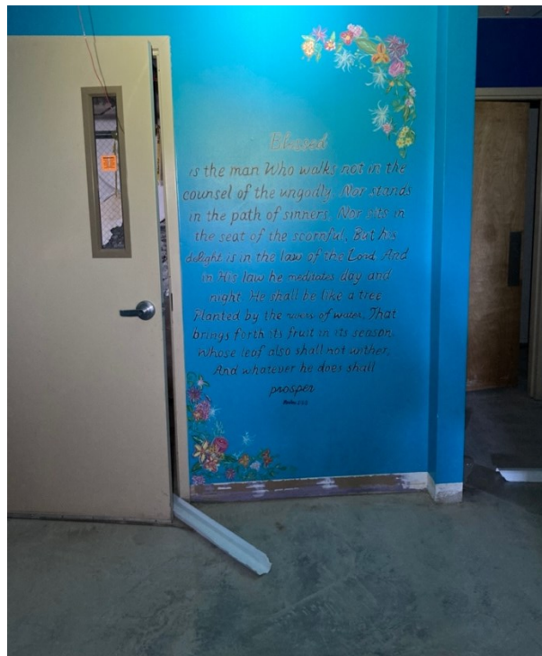
Figure 34: "Site-Work, basement mural intact surrounded by broken infrastructure." March 2024
