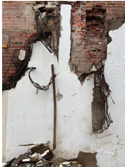
Figure 66: “Site-Work, documentation of deterioration.” March 2024
