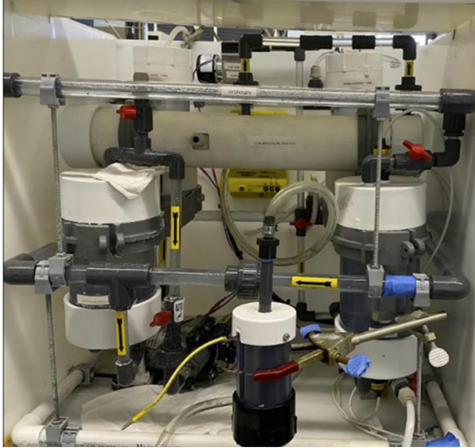
Figure 3-7: MMP Unit 1 (Hypochlorous acid generator)
