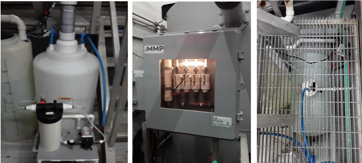
Figure 22. MMP Dirigo Stream Unit and buffer tank at Biddeford Pool Plant.
