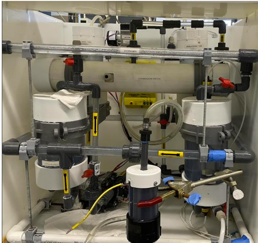
Figure 1. MMP Unit (Hypochlorous acid generator)
