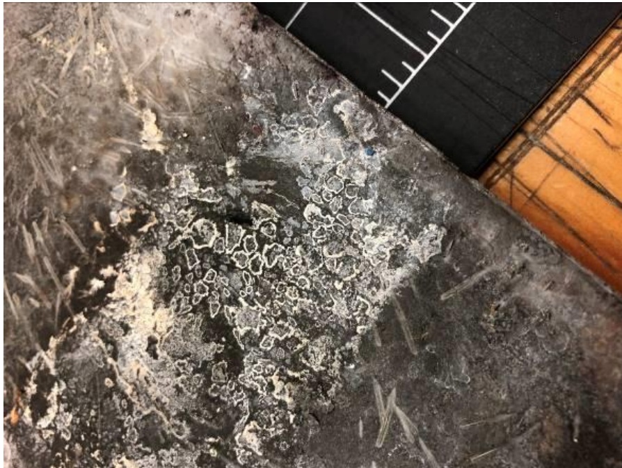
Figure 3.8. White residue on UHPC surface
