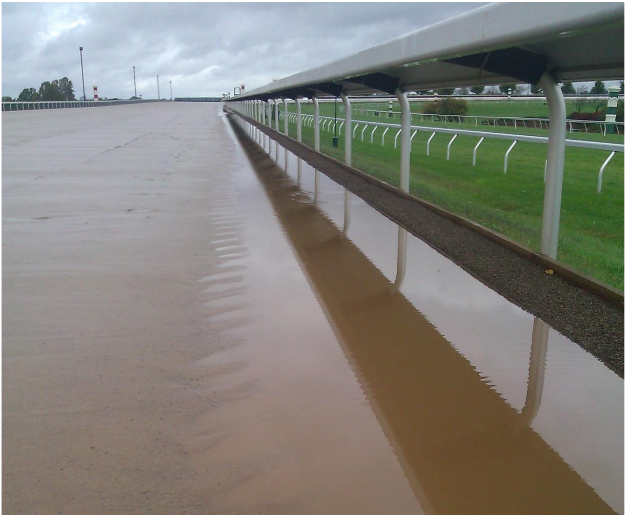
Figure 15: Standing water on a track that has been saturated by rainfall.
