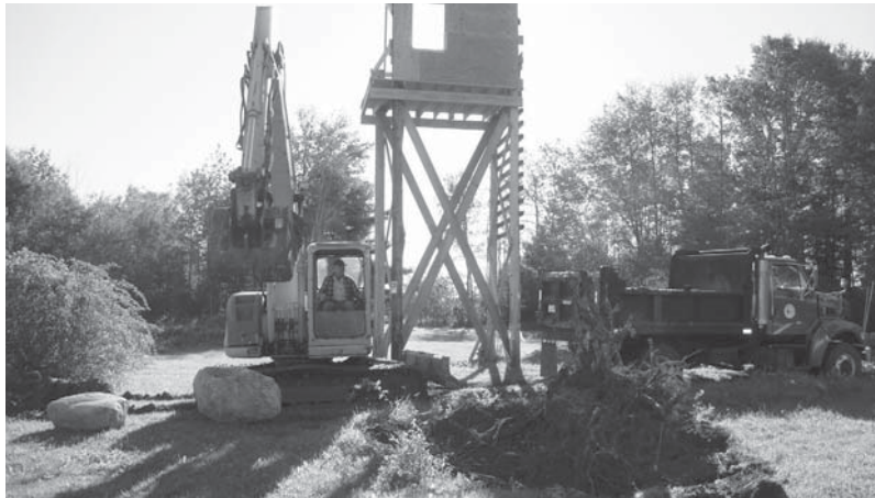
Merton Moore dredging the fire pond with help from the road crew
