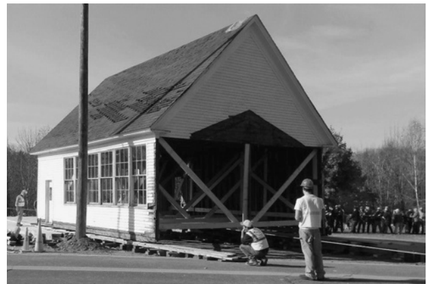
The Lincolnville Community Library opened on February 1, 2014, in this renovated one-room schoolhouse built originally in 1849. The opening date was just 15 months after nearly 200 community members helped pull the old building across Main Street to a formerly vacant lot (seen here). A large team of skilled volunteers and professional contractors worked together to turn the old schoolhouse into Lincolnville’s new library. (Photo courtesy of Lincolnville Community Library)
