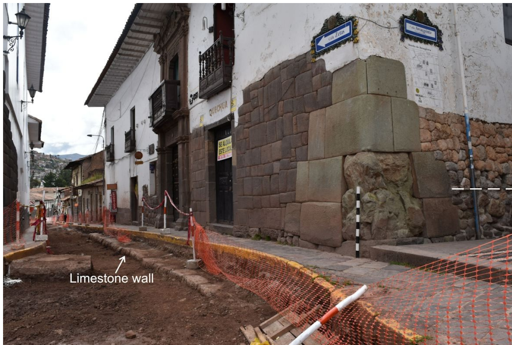
Figure 15. Stone terrace wall that formed part of the exterior of the Qoricancha.
