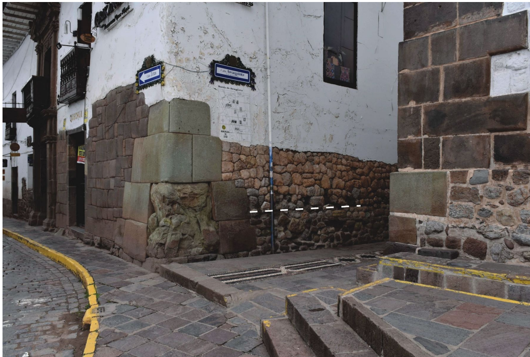
Figure 13. The corner of Awaq̄pinta Street with a green diorite veneer. The dotted line marks the original street level. Below it the foundation can be seen. The green diorite corner on the right must have been demolished when the Santo Domingo monastery was built over the Qoricancha .
