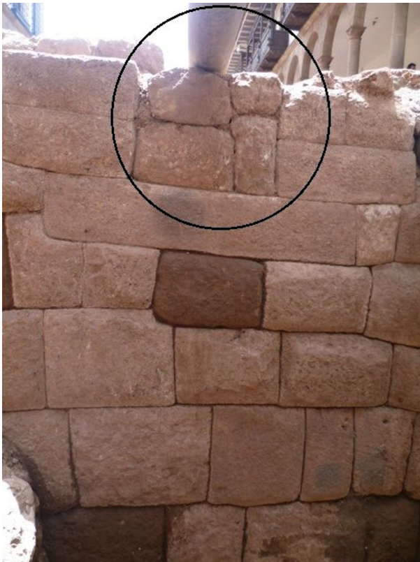
Figure 29. Detail of the blockage of the Inca wall canal.
