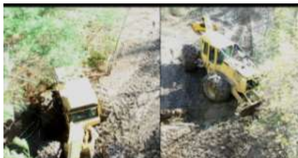
Fig. 1: Skidder installing water bar. Left, facing downslope. Right, facing upslope. Note skidder's rear tires remain on trail.
