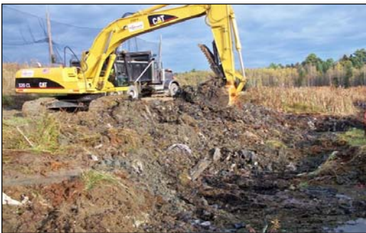
Area 1 remediation removing waste that is outside the closed cap of the landfill
