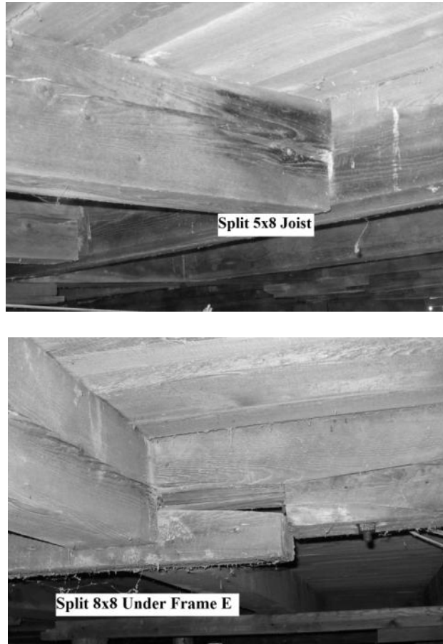
Figure 14: Issues with Floor Framing
